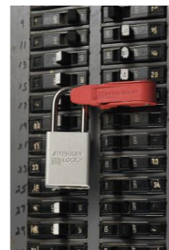
Circuit Breaker Lockout
